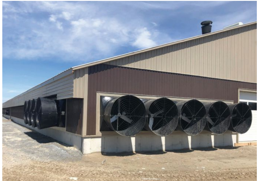
Be sure to wash or clean fan housings and shutters of any dirt or debris to ensure optimal performance.
